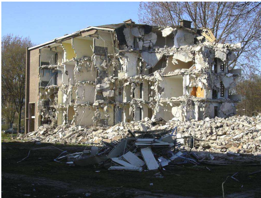
Figure 1. Many buildings are demolished and end up as landfill, because they do not meet today's standards for usage, and because they are not designed for disassembly and reuse.
