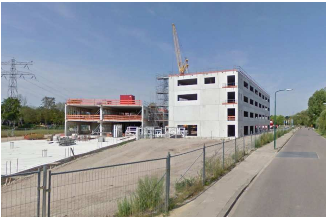
Figure 15. Construction of the school, summer 2009 (almost same point of view as figure 14).
